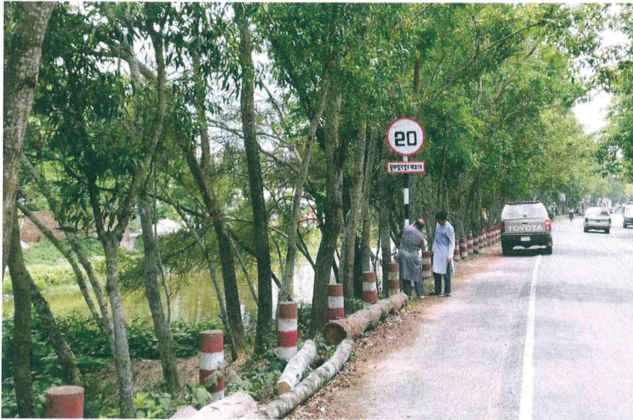
Figure 06a: Unspecified Speed Limit Sign (Near LRP 019)
