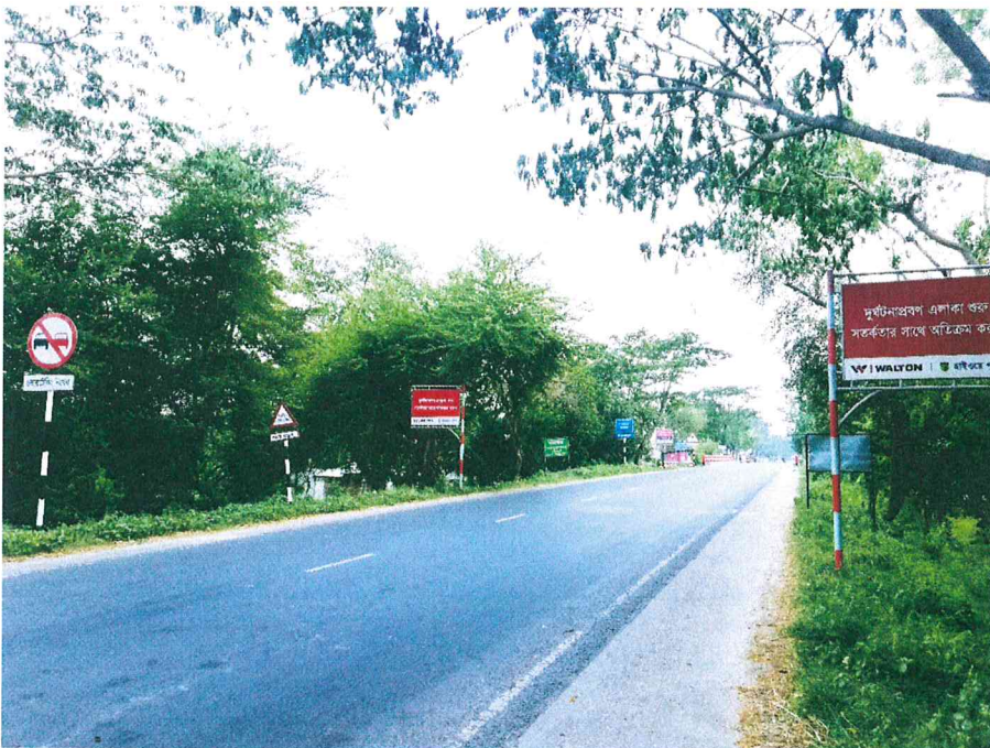
Figure 06b: Incorrect Road Marking at No Overtaking Area (Near LRP 108)
